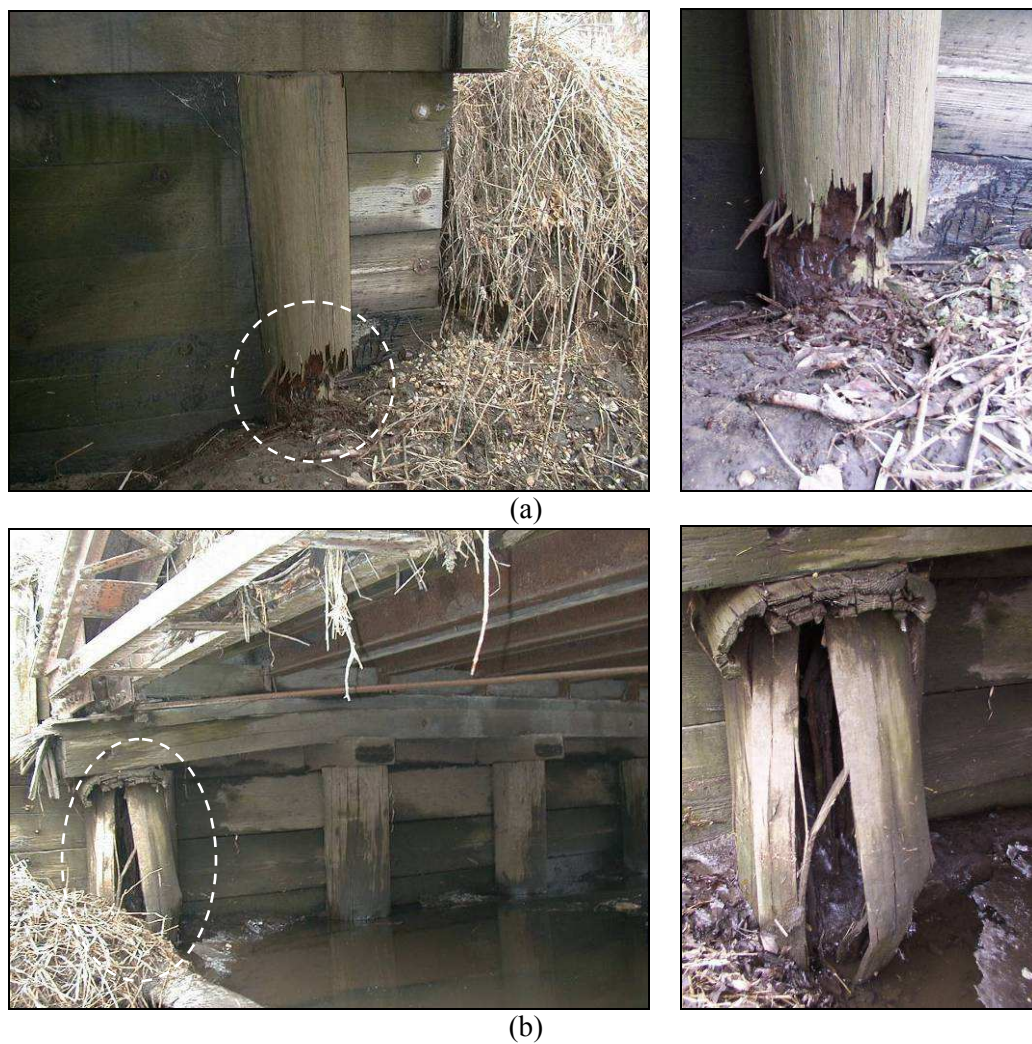
FIG. 4.1 — Timber pile biological deterioration (a) reduction of pile cross section (b) complete deterioration of pile section
