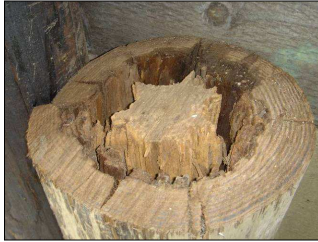
FIG. 4.6 — Internal pile deterioration that is difficult to detected using the stress wave technique
