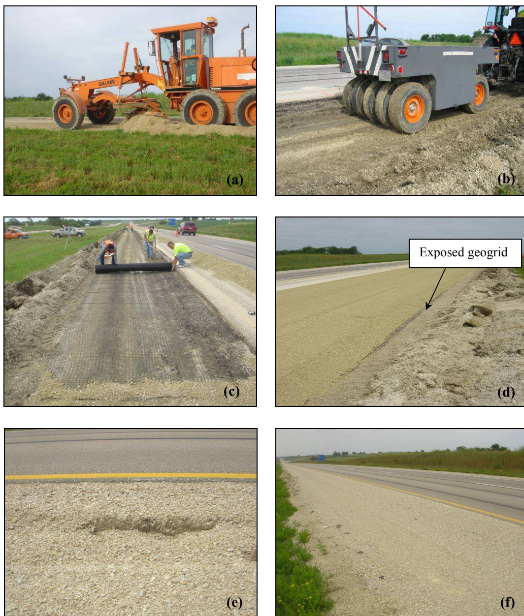
FIG. 3.5 — Shoulder reconstruction using geogrids (a) motor grader removing the contaminated granular layer (b) pneumatic roller used to compact the subgrade (c) rolling the geogrid over the subgrade (d) spreading the aggregate over the geogrid (e) rutting developed at the control section after one month (f) no rutting at the geogrid stabilized section after one month
